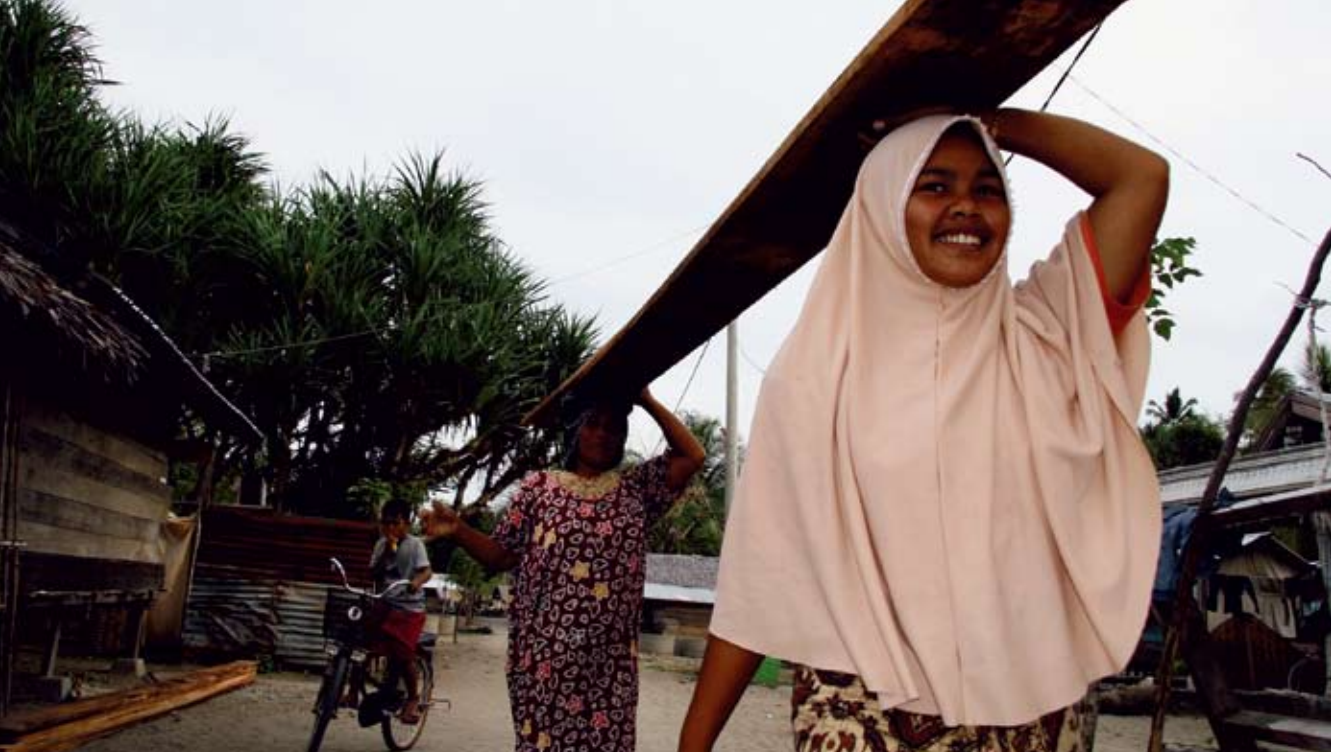
Rebuilding after the destruction wrought by a tsunami killer wave in Banda Aceh, Indonesia. Photo © UN-HABITAT
