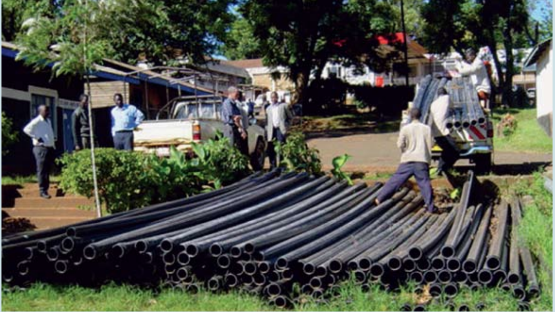
Contractor delivering pipes for a water project in Kisii, Kenya. Photo © UN-HABITAT
