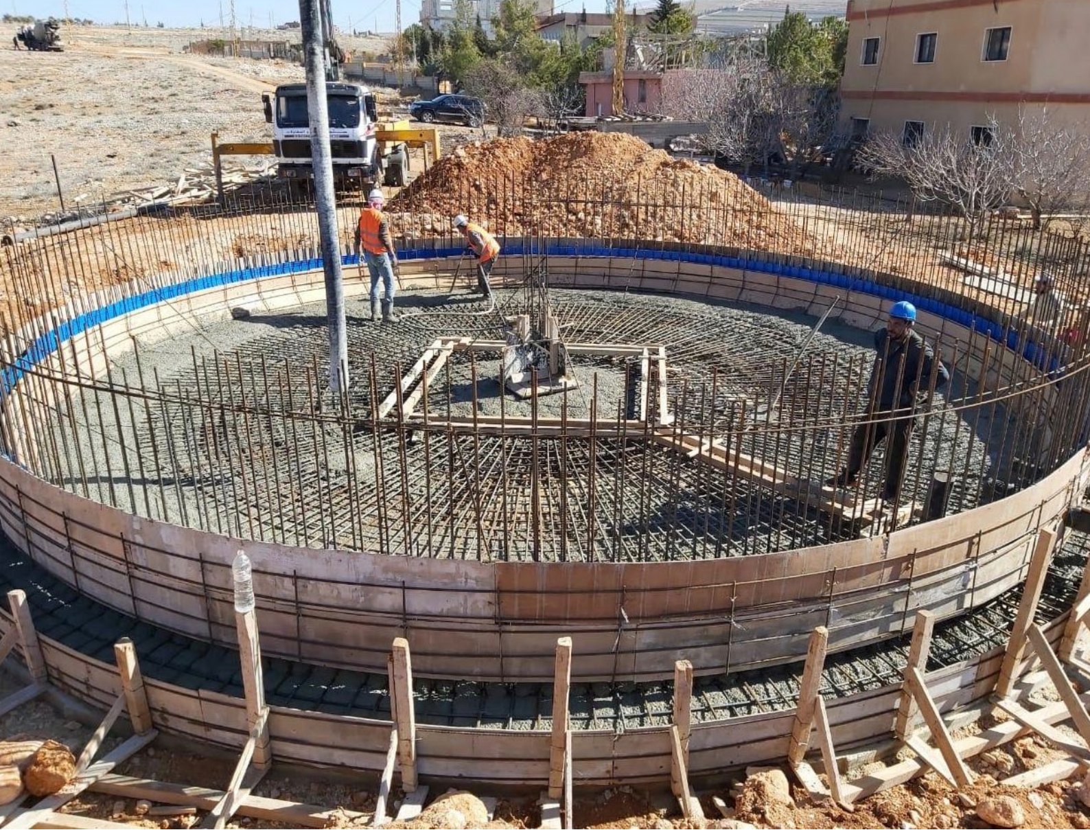
A view at the construction of a well as part of the project of ADRA Slovakia and ADRA Lebanon, supported by SlovakAid.
