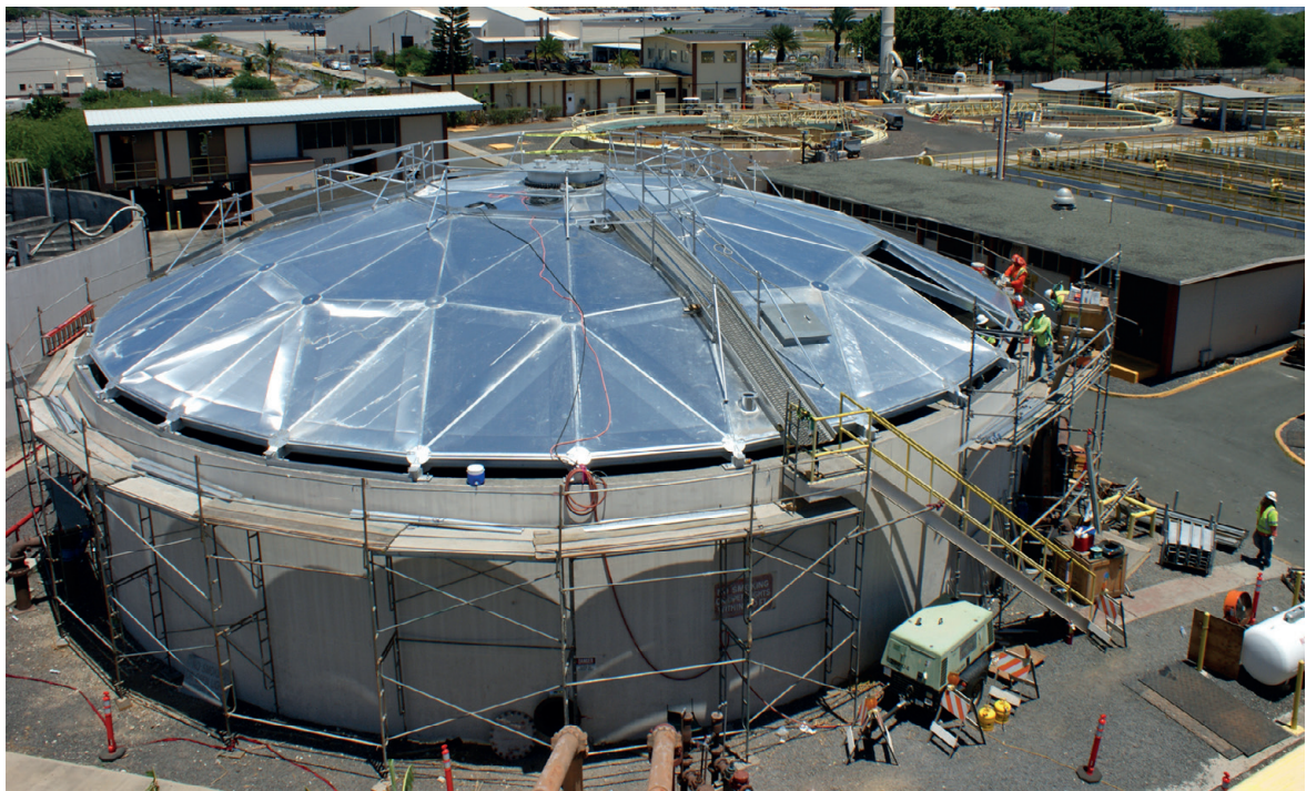
The wastewater treatment plant at the US military's Joint Base Pearl Harbor-Hickam has been retrofitted to capture methane gas for future energy use. Photo: Flickr / US Navy / Denise Emsley
