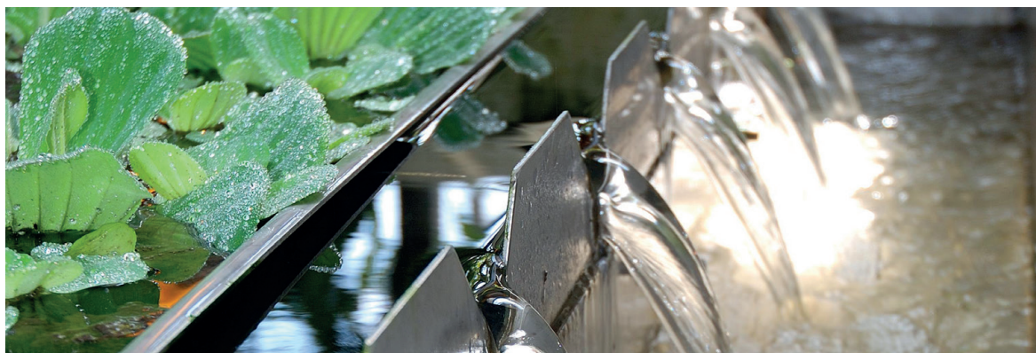
Part of a low-energy wastewater treatment system based around a cascade of biological stages. Biofilms of microorganisms, some living on plant roots, remove nutrients from the effluent. Photo: Organica
