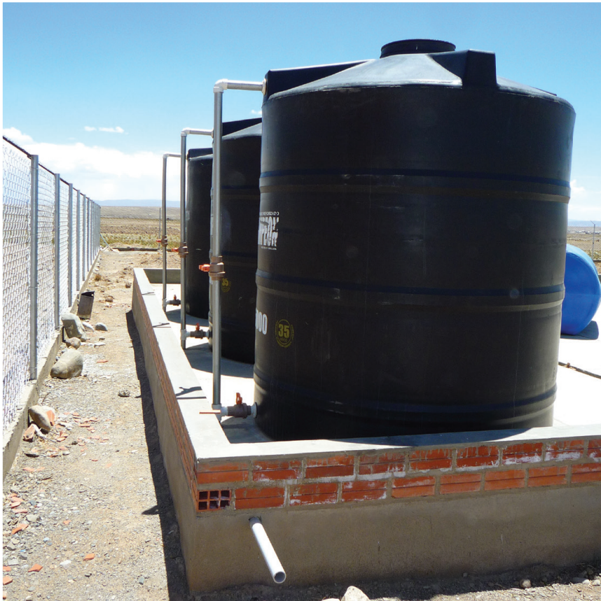
Storage tanks for source-separated urine, El Alto, Bolivia. Photo: Kim Andersson
