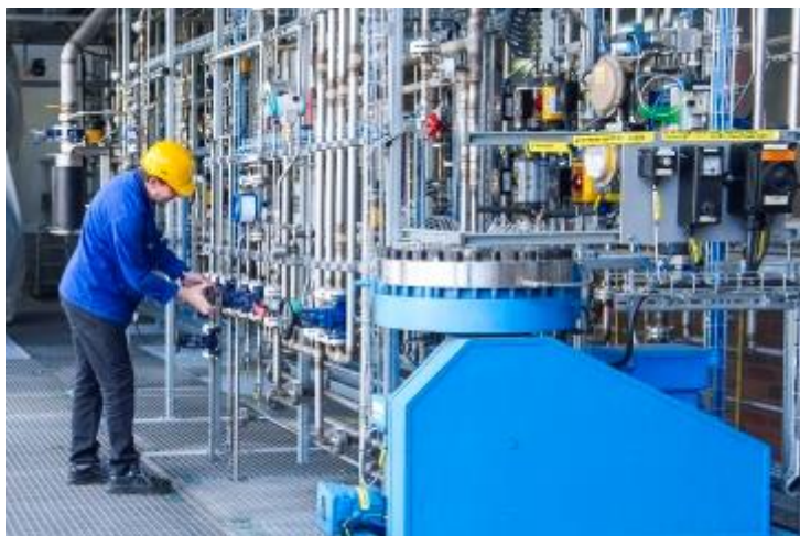
Methane pyrolysis for CO 2 -free hydrogen
