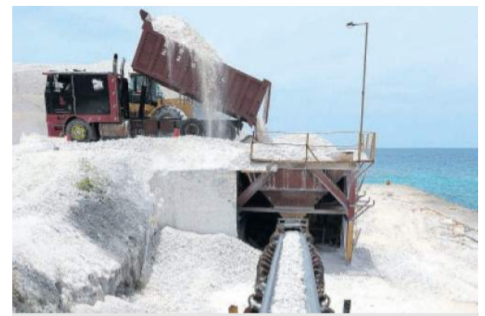
A truck dumps limestone into the conveyor system at Lydford Mining Limited, a major player in the limestone industry.
