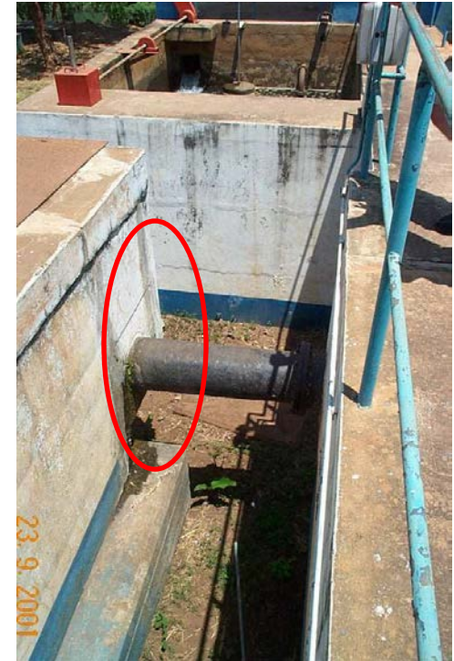
Cracks and leaks from a rigid connection
