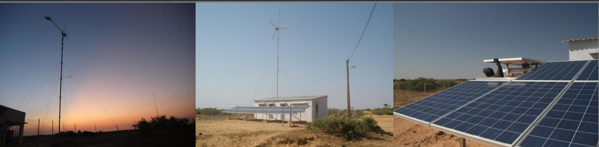
Foto: Wind-Solar-Diesel hybrid power system with battery storage for village power supply designed and operated by ENERSA S.A., Senegal; INENSUS
