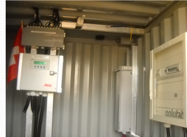
Regulator – Inverter– Distribution board
