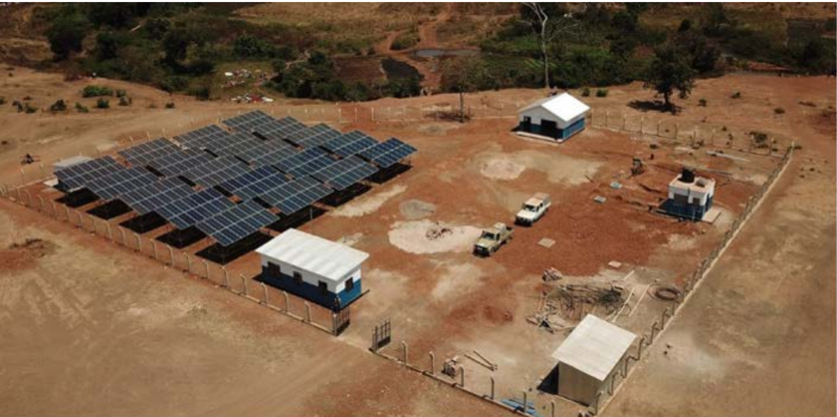
Figure 6. Solar pumping system installed in a refugee camp in Tanzania (Source:Water Mission)
