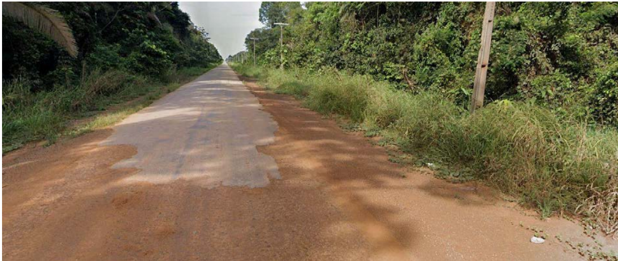
Figure 47. End of the asphalt (in 2024) of the BR-319 highway Manaus – Porto Velho, at the southern End of the “Trecho do Meio”, ca. 25 km north of the BR-230 and BR-319 turnoff
