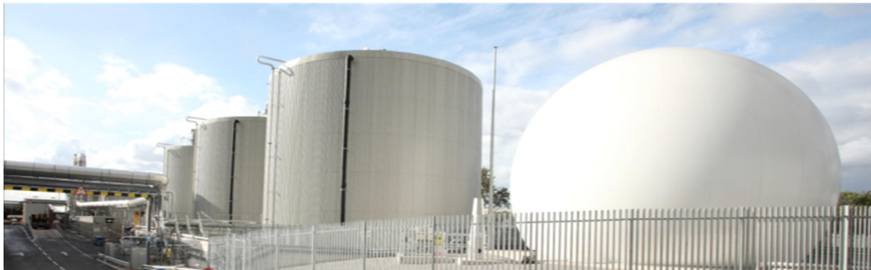
Anaerobic digestion facility
