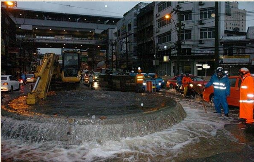
Bangkok flood by pipe broken on 16 Oct 2013
