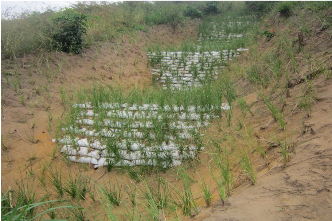
Urban gully erosion stabilized with vetiver grass in Kimwenda, on the outskirts of Kinshasa
