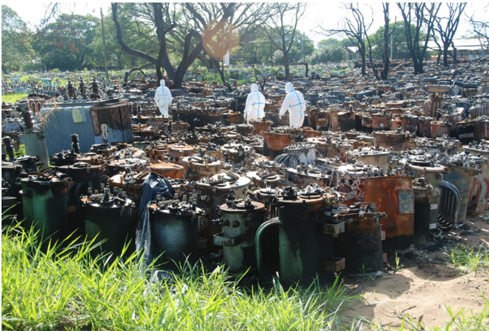
Electrical equipment damaged by fire outside Asuncion, Paraguay
