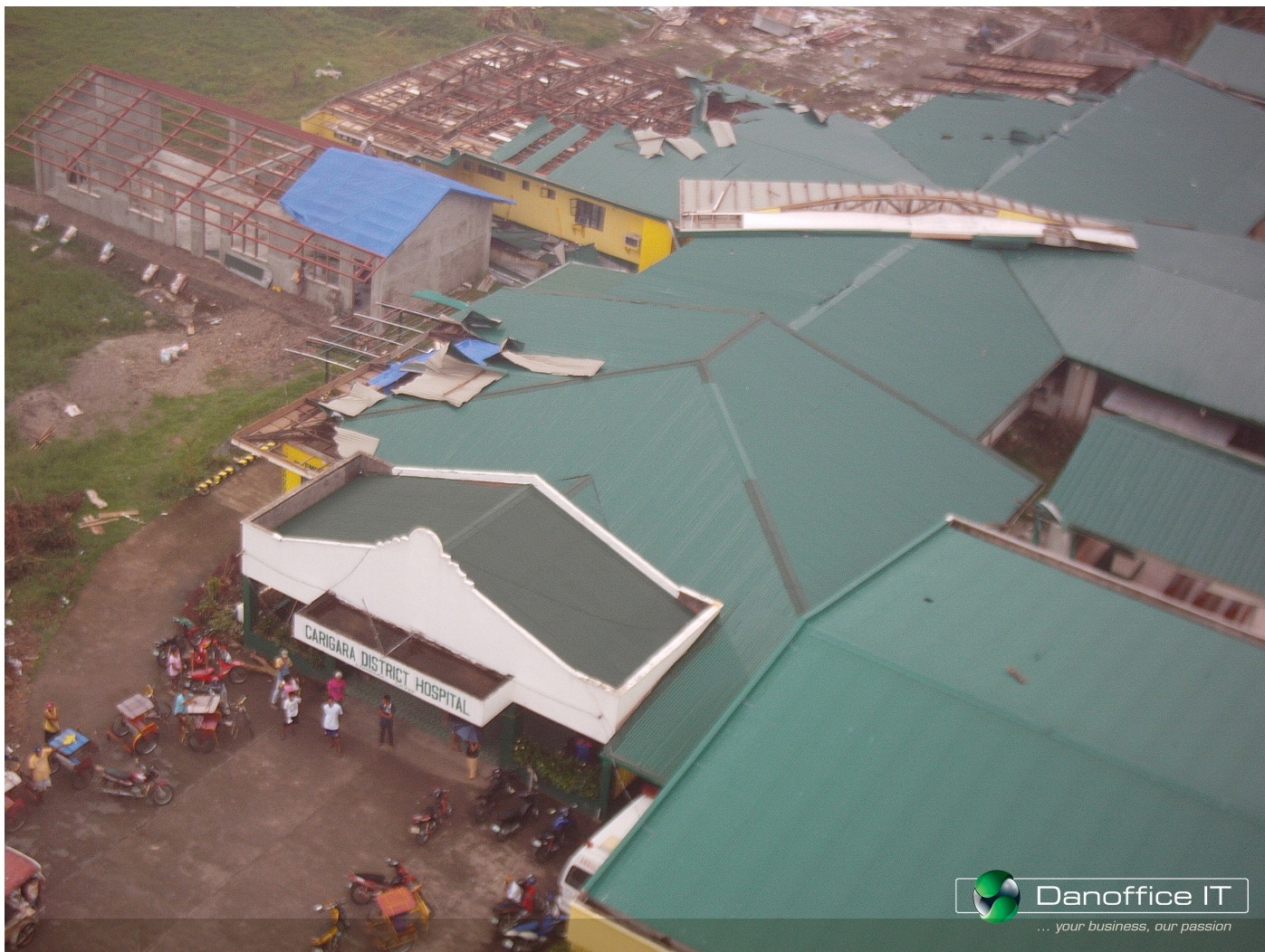
Figure 2 An image from above, taken by the quadcopter drone that was provided by Danoffice IT in support of the humanitarian response in The Philippines. The drone was used to survey damage of the Carigara Hospital in typhoon-hit Tacloban in November 2013.
