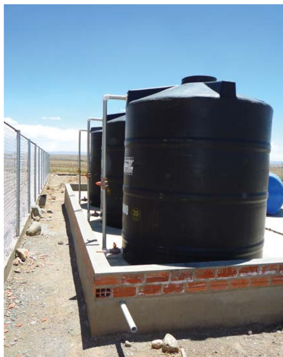
Storage tanks for source-separated urine, El Alto, Bolivia. Photo: Kim Andersson
