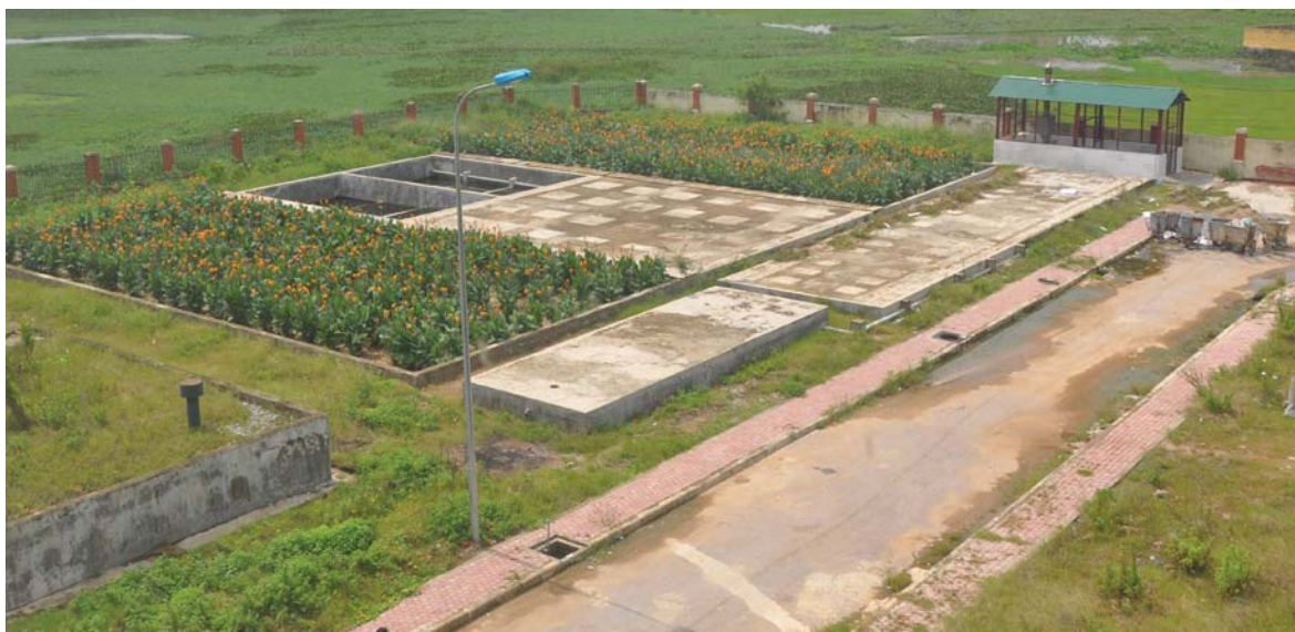
Decentralized plant treating hospital wastewater, Thanh Hóa, Vietnam. Photo: Flickr /frapoberlin
