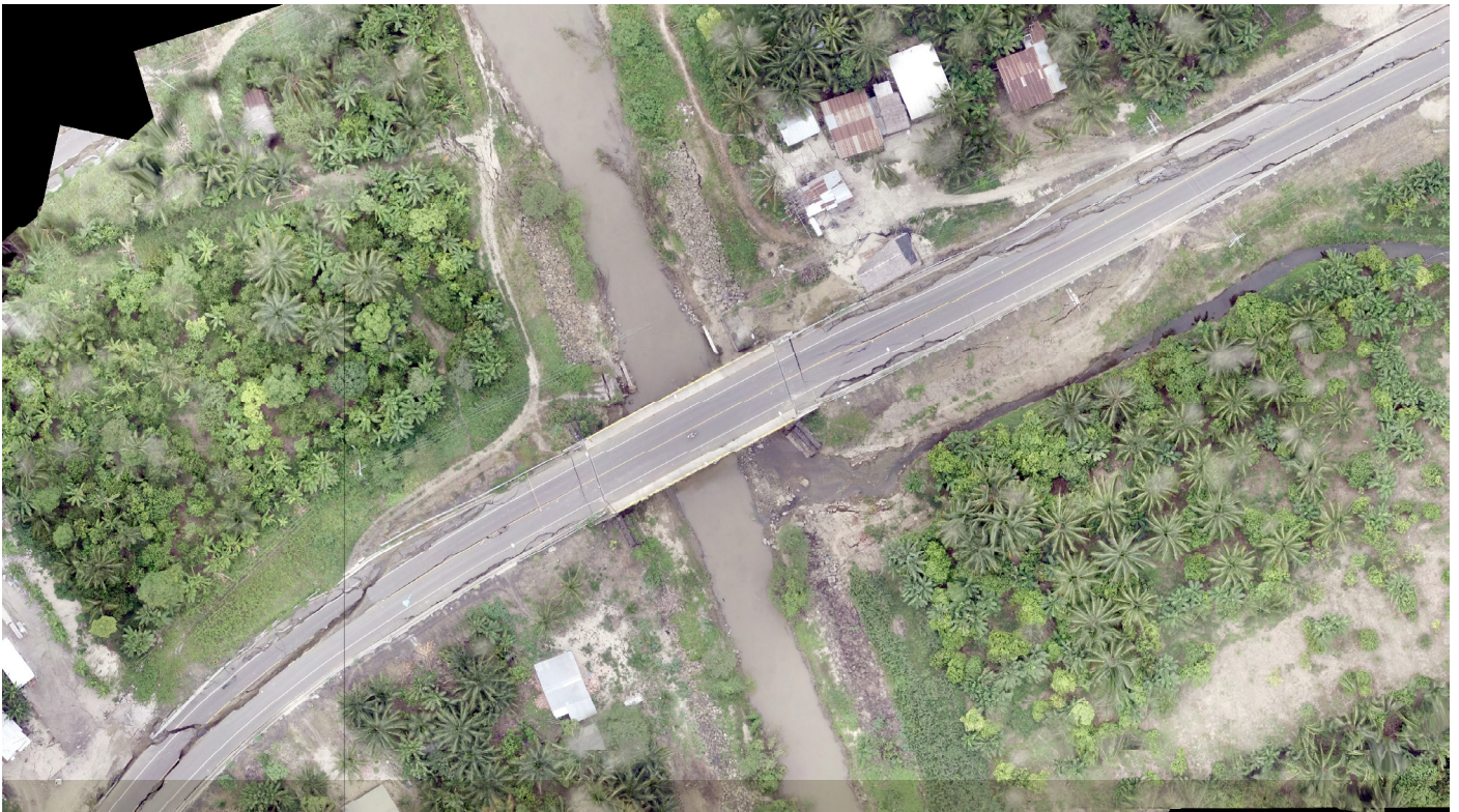
Figure 5 Aerial imaging of a damaged bridge taken by a Phantom 3 pro on a flight conducted together with the Ecuador Ministry of Transport. Francisco Ruiz, April 2016.
