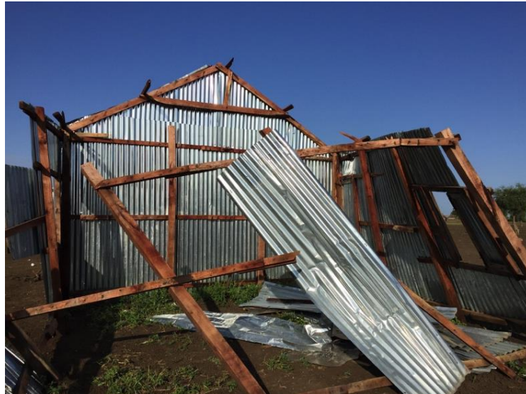
Figure 9 Wind & Rain Damage to Wad As Saboor Mixed School, Al Mafaza.
