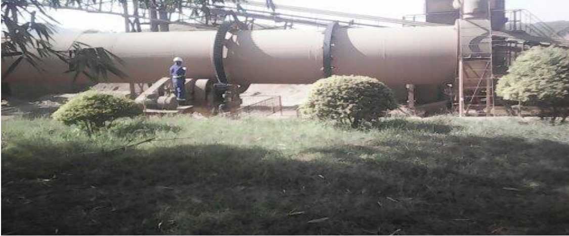
A Worker in engineering section repairing the kiln full PPEs (full compliance to safety)
