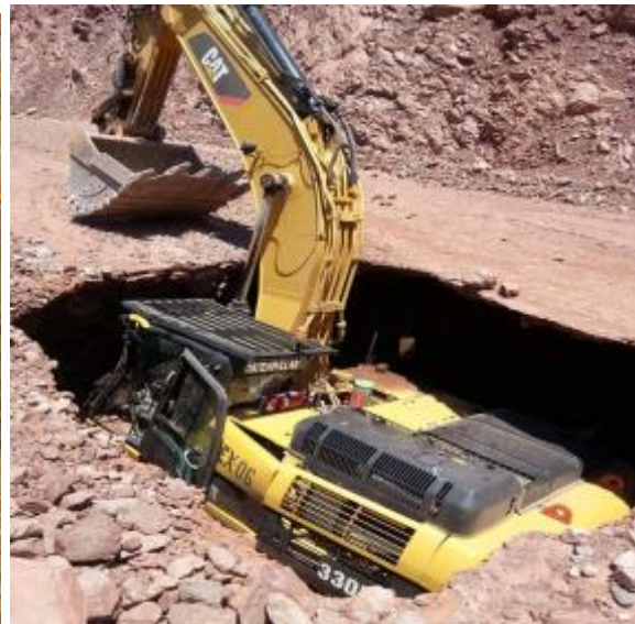
excavator sank into non-consolidated surface Namekara mine
