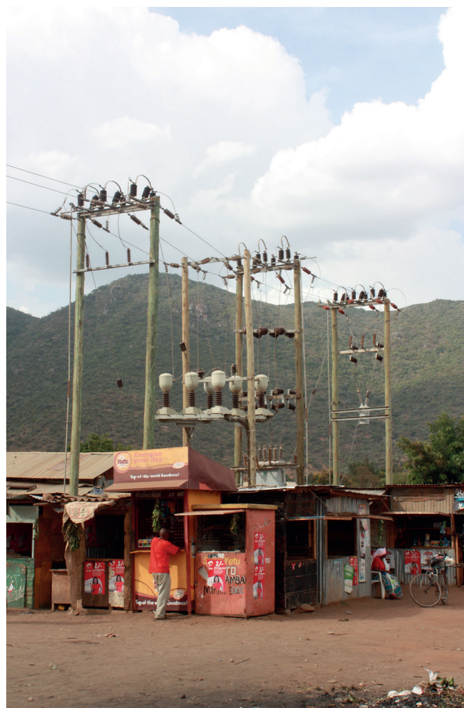
An electrical distribution and transmission project in rural Kenya, where electrical coverage remains low
