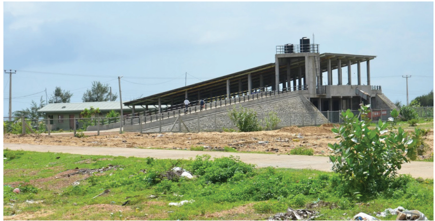
Composting plant in Ampara District built under ERP-I
