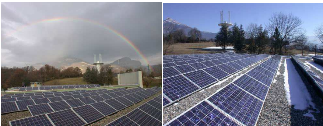
Figure 25. Perspective of existing state of the art flat roof mounted PV systems 4
