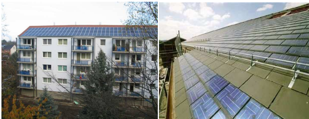
Figure 29. Perspective of existing state of the art “standard in-roof” systems (left image) and solar shingles or tiles
